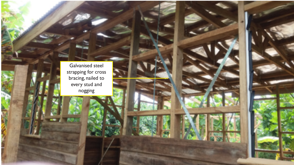
Figure A16: Stud frame wall with galvanised steel strap bracing (Source: Fiji Rural Housing Unit)
